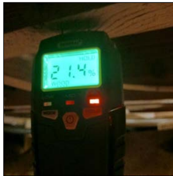
High moisture levels
