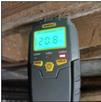
High moisture levels
