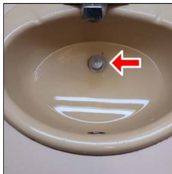
Master sink slow drain
