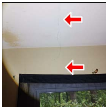
Displaced drywall cracks throughout
