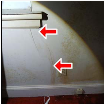
Displaced drywall cracks throughout
