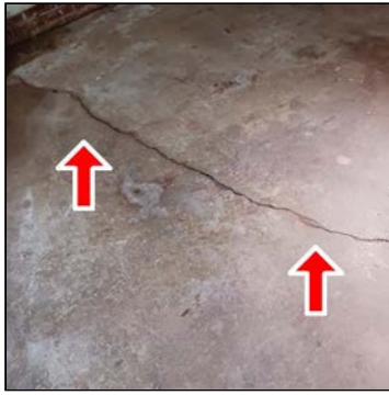
Garage slab cracks
