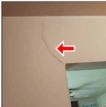
Displaced drywall cracks throughout
