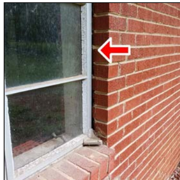
Front left window gap
