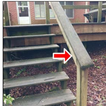
Rear deck step railing loose
