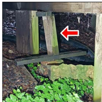
Missing column footings
