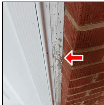
Possible lead based paint
