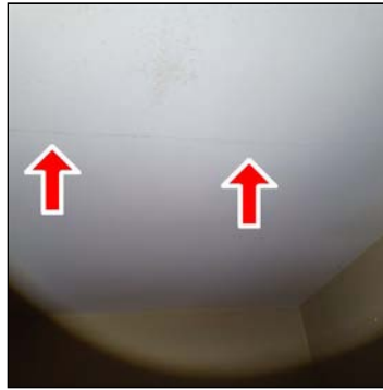
Displaced drywall cracks throughout
