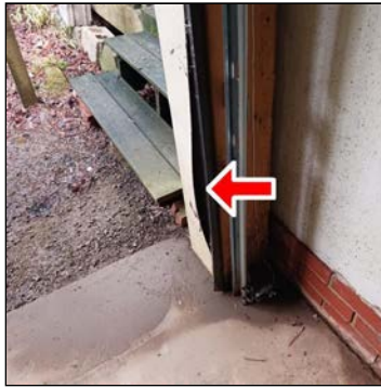
Loose trim around garage door
