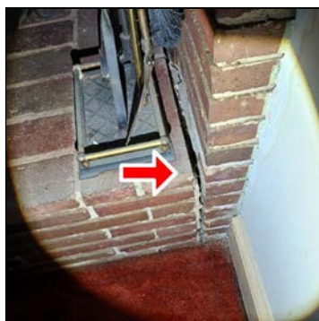
Large gaps at base of fireplace
