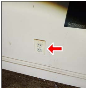
Ungrounded outlets throughout
