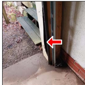
Loose trim around garage door
