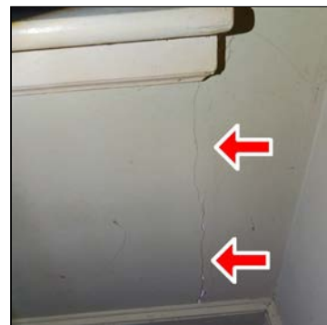
Displaced drywall cracks throughout
