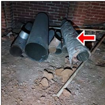
Trash in crawl space
