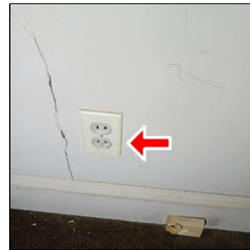
Ungrounded outlets throughout
