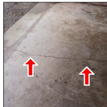
Garage slab cracks
