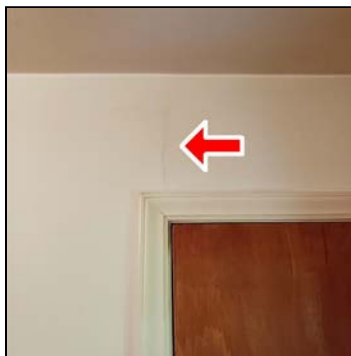
Displaced drywall cracks throughout
