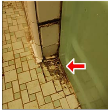
Damaged floor hall bathroom
