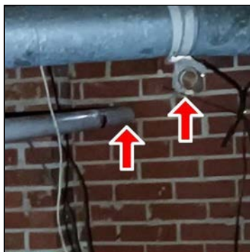
Furnace flue vent disconnected in crawl
