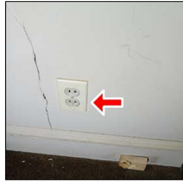
Ungrounded outlets throughout
