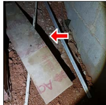
Trash in crawl space
