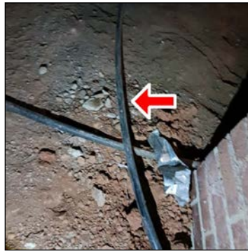
Trash in crawl space
