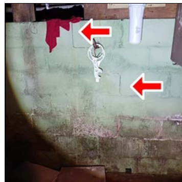
Basement wall crack
