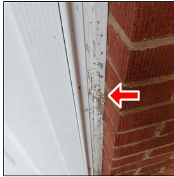
Possible lead based paint
