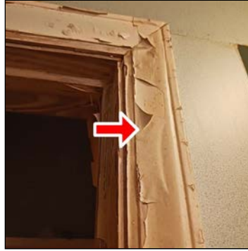
Possible lead based paint
