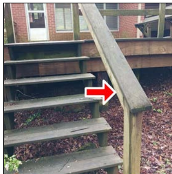
Rear deck step railing loose
