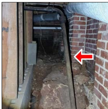
Cast iron pipes
