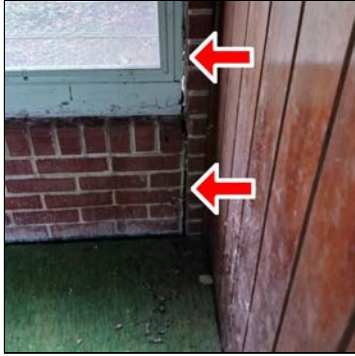
Visible daylight in garage walkway walls
