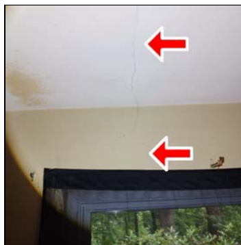
Displaced drywall cracks throughout
