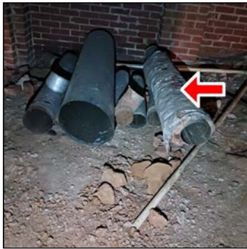
Trash in crawl space
