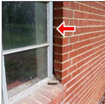
Front left window gap
