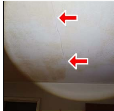
Displaced drywall cracks throughout
