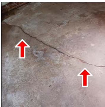
Garage slab cracks
