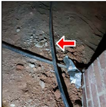
Trash in crawl space
