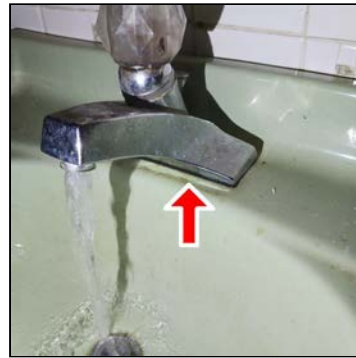
Hall bath sink leaks
