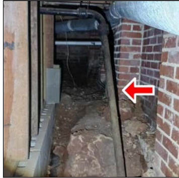
Cast iron pipes
