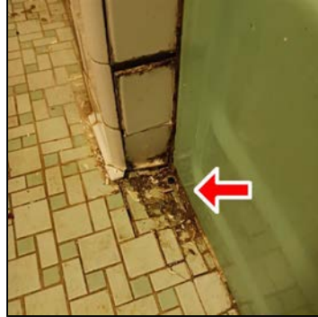
Damaged floor hall bathroom
