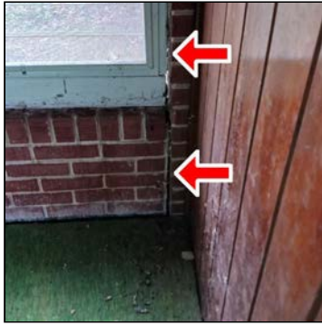
Visible daylight in garage walkway walls
