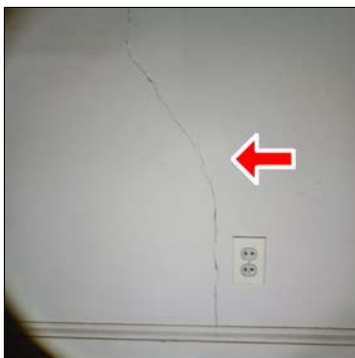
Displaced drywall cracks throughout
