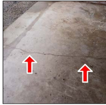
Garage slab cracks
