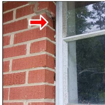
Front left window gap
