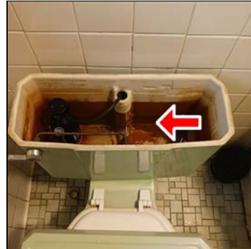
Hall bath toilet
