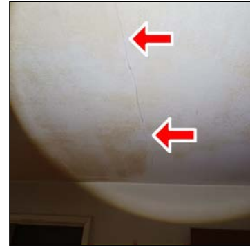
Displaced drywall cracks throughout
