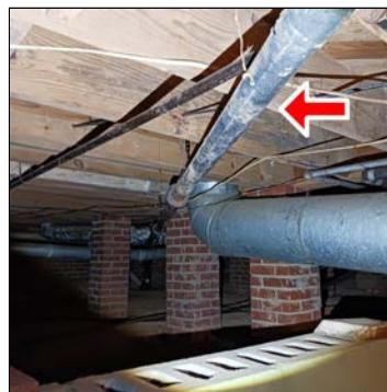
Cast iron pipes
