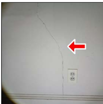
Displaced drywall cracks throughout
