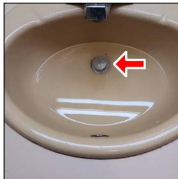
Master sink slow drain
