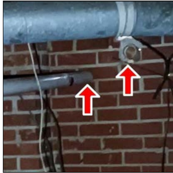
Furnace flue vent disconnected in crawl
