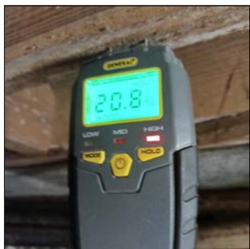
High moisture levels
