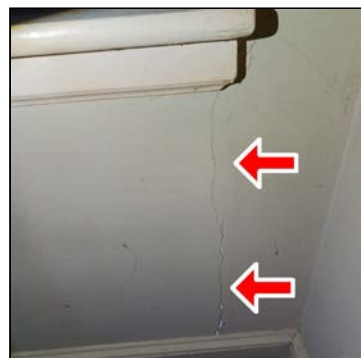
Displaced drywall cracks throughout
