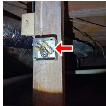
Missing junction box cover in crawl
