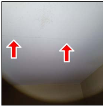
Displaced drywall cracks throughout
