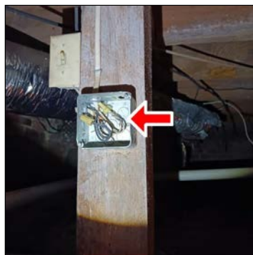
Missing junction box cover in crawl
