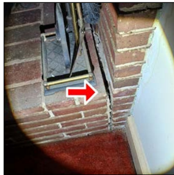
Large gaps at base of fireplace
