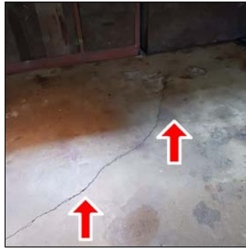
Garage slab cracks
