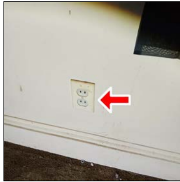
Ungrounded outlets throughout
