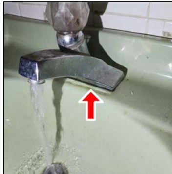
Hall bath sink leaks
