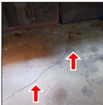
Garage slab cracks
