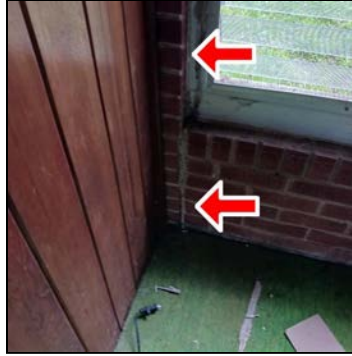
Visible daylight in garage walkway walls
