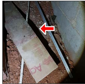
Trash in crawl space
