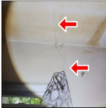
Displaced drywall cracks throughout
