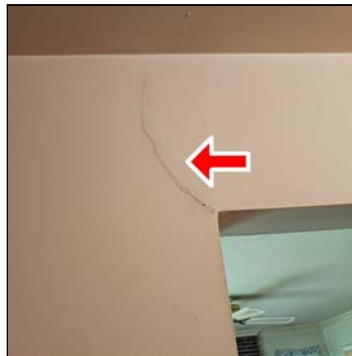
Displaced drywall cracks throughout
