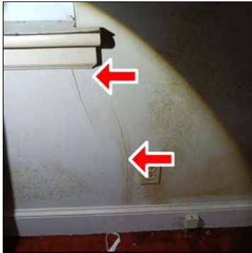
Displaced drywall cracks throughout
