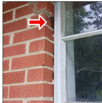
Front left window gap
