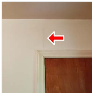
Displaced drywall cracks throughout
