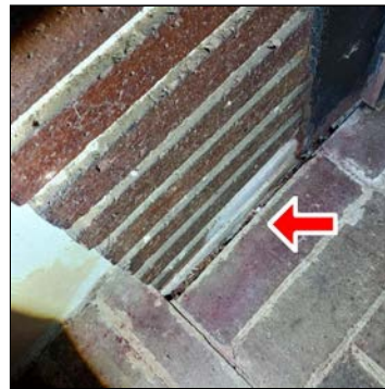
Large gaps at base of fireplace
