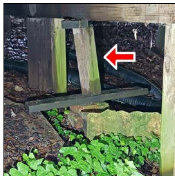
Missing column footings
