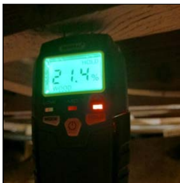
High moisture levels
