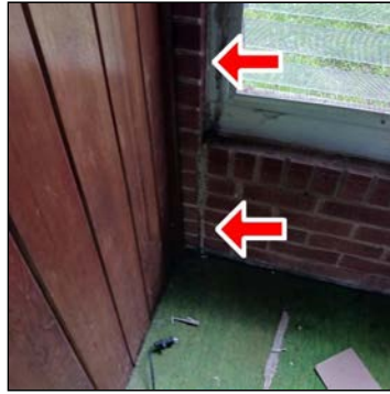
Visible daylight in garage walkway walls
