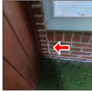
Visible daylight in garage walkway walls
