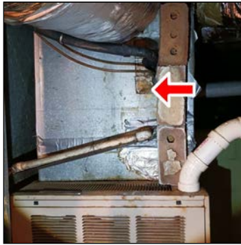
Indoor coil not inspected
