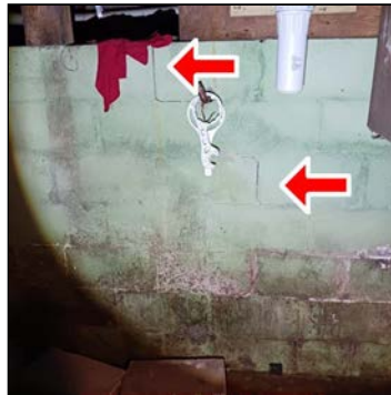
Basement wall crack
