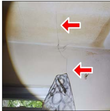
Displaced drywall cracks throughout
