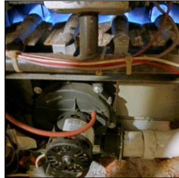
Furnace burners on
