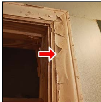
Possible lead based paint
