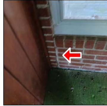
Visible daylight in garage walkway walls
